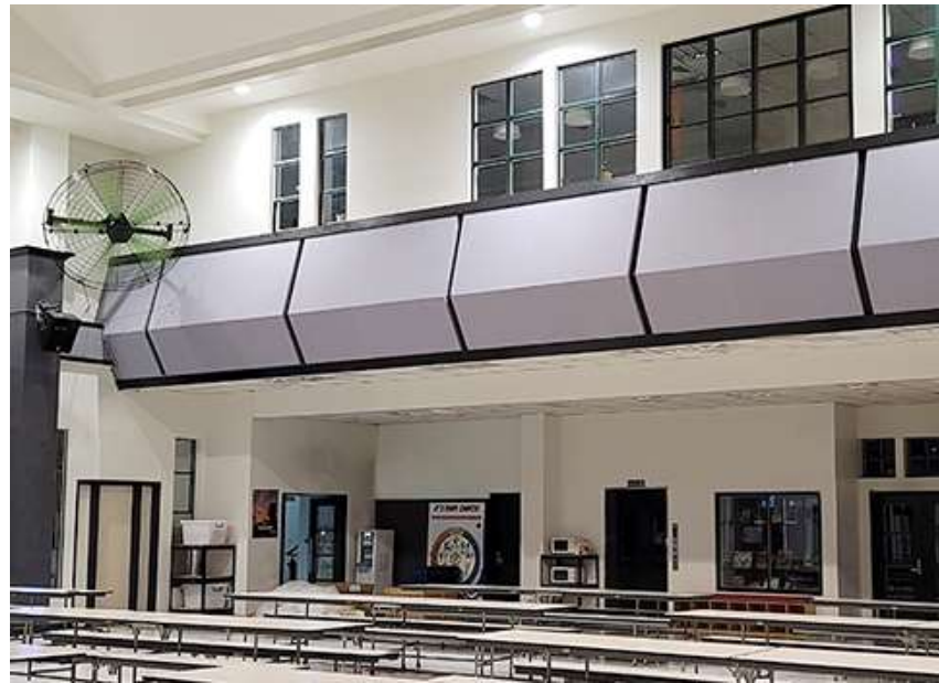
Taiwan / School Hall Wall-Mount Fan
