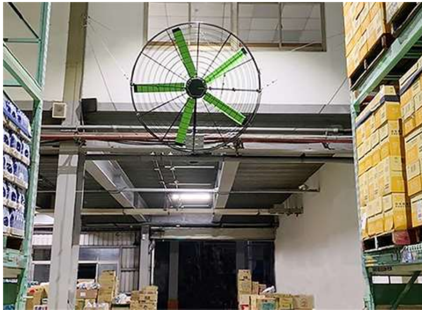
Taiwan / Factory Wall-Mount Fan
